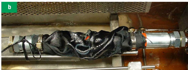
Fig. 2 - (a) Before the burst; (b) after the burst.
